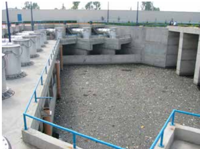
Figure 1: A wastewater sump covered with floating debris.
